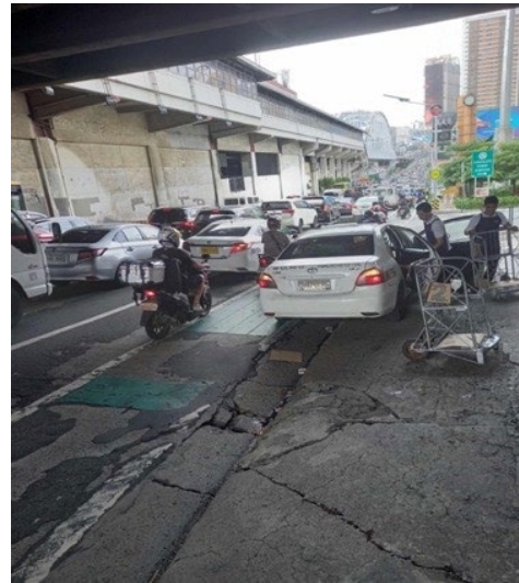
Figure 11: A most senior age group participant often passed through this area with damaged pavement and would trip.
